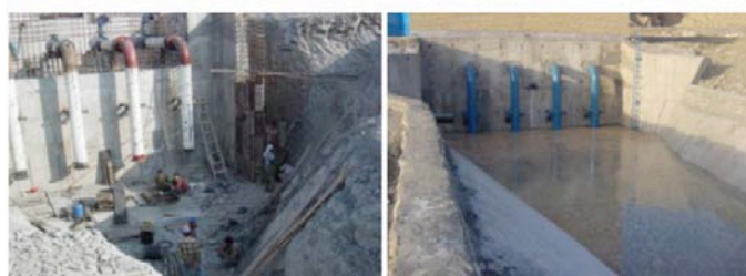
Emergency pumping station (bottom) to exploit dead storage of the Minab Dam (Top) located in Hormozgan Province (Southern Iran)
