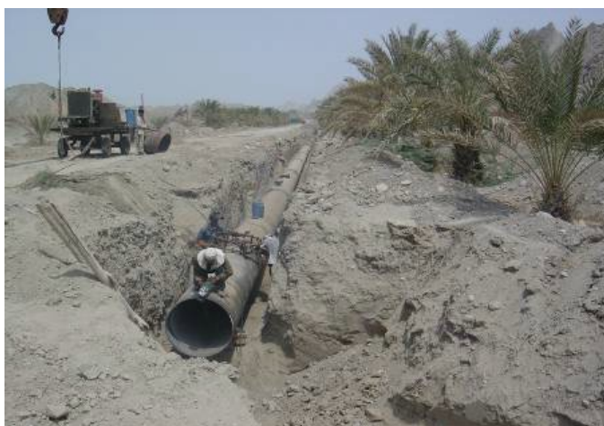
The Sistan Emergency pipeline from Chanimeh reservoir to 600 villages (South-eastern Iran)
